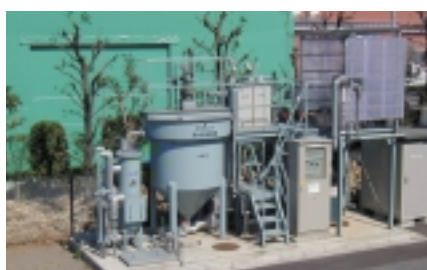
Wastewater treatment facilities
